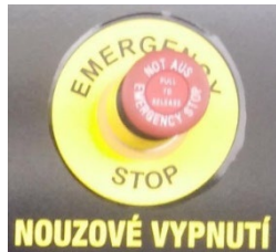
Emergency shutdown button (ESD)
